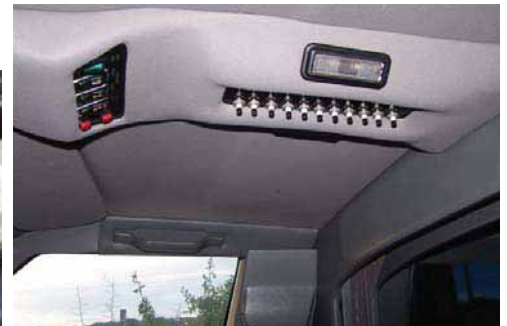
“More circuit breakers than a 747”
